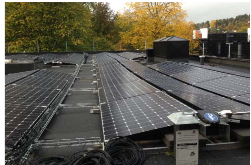
PV on roof (block 4). Photo: Skanska
