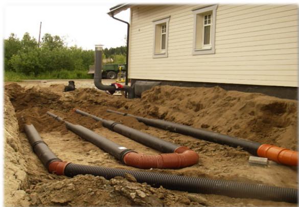
Figure 27 NorOne ground heat exchanger, ID 250 mm, 50 m ( www.norone.info )
