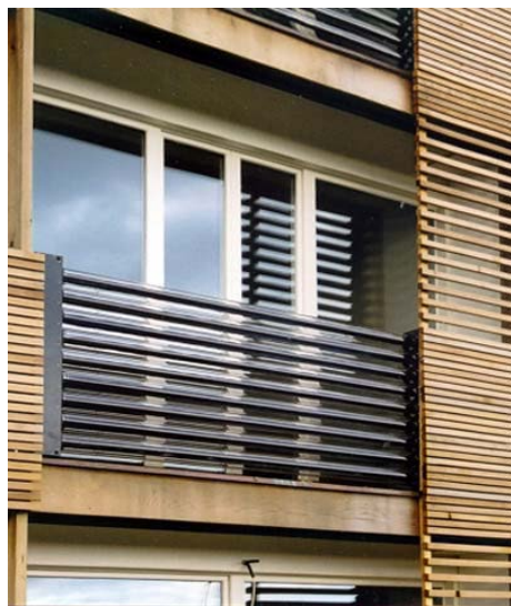
Vacuum solar thermal collectors in rows on balcony, apt. Block, Zürich. Source: Robert Hastings
